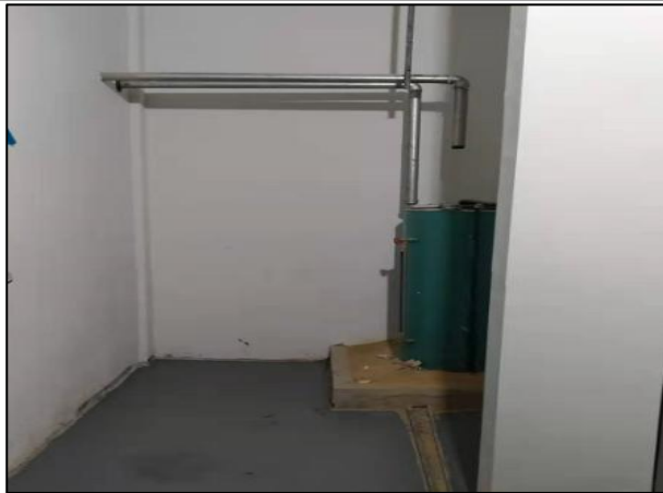
3B地块储油罐
